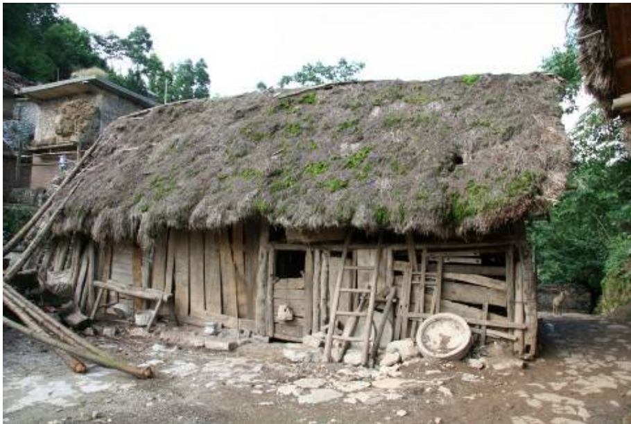
Fig. 11 some local people's houses are purely made of wood and grass, without any renovations
